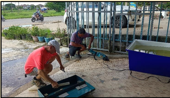
The low water pressure for 4 months has been fixed.
