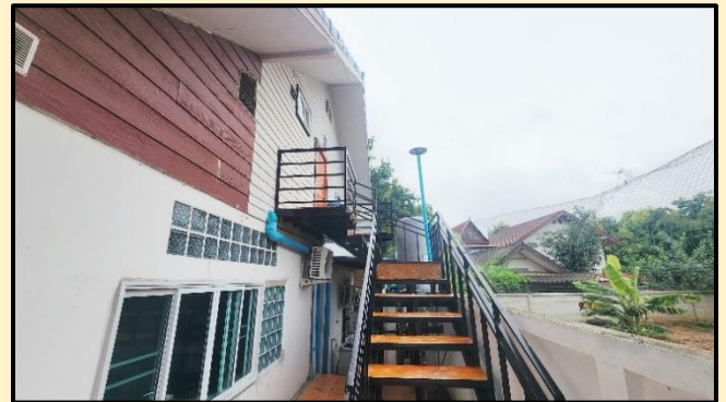
We need to add a covering to the second floor entry.
