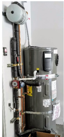
H.P water heater
