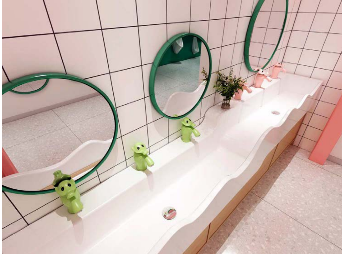
KINDERGARTEN WASHBASIN INDICATION
