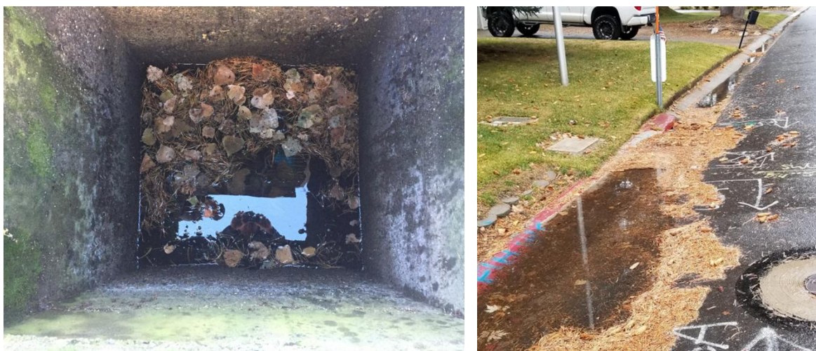
Figure 2. Examples of Debris Buildup at Storm Drains within Tahoe Keys
