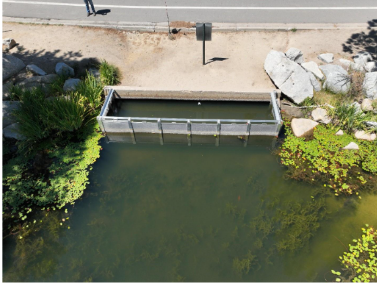
Figure 14. The 15 th Street screening system.
