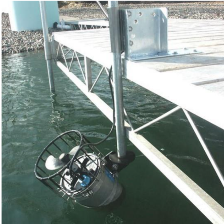
Figure 68. Example of a dock bubbler
