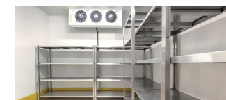
RESTAURANT COLD ROOMS
