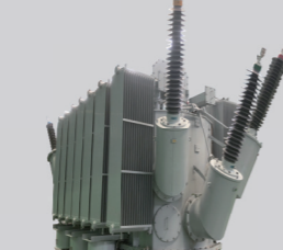
110kV Mobile Transformer
