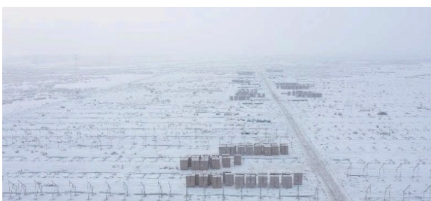
Xinjiang Lixin 37.5MW/150MWh Energy Storage Project SC(B)-2750/37kV Cast Resin Dry Type Transformer
