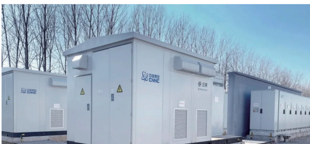
Tancheng 101MW/204MWh Energy Storage Project SC(B)-3750/37kV Cast Resin Dry Type Transformer
