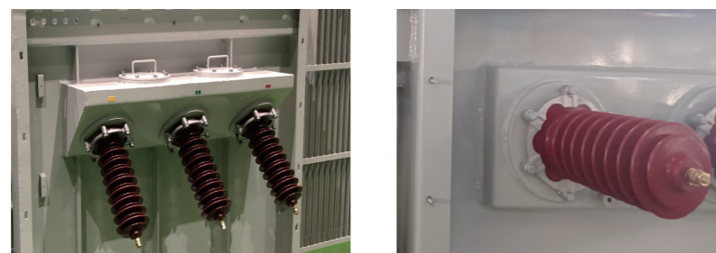
hand hole structure
