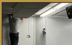
New PTZ Camera installed
