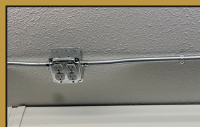
Electrical outlet installed
