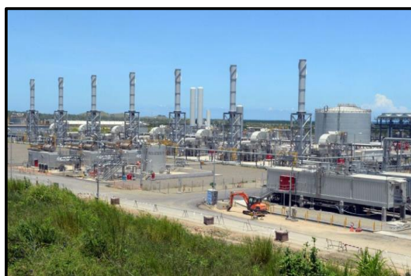
A liquid natural gas facility in Port Moresby
