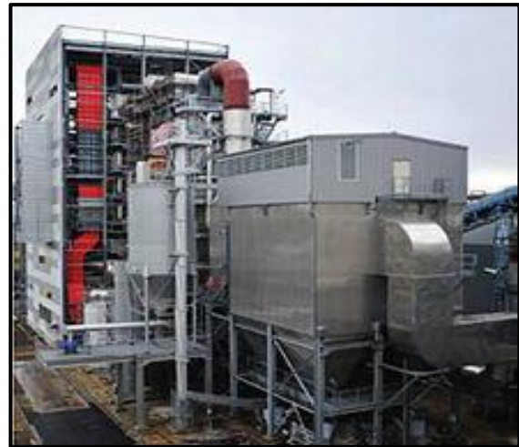
A biomass energy station
