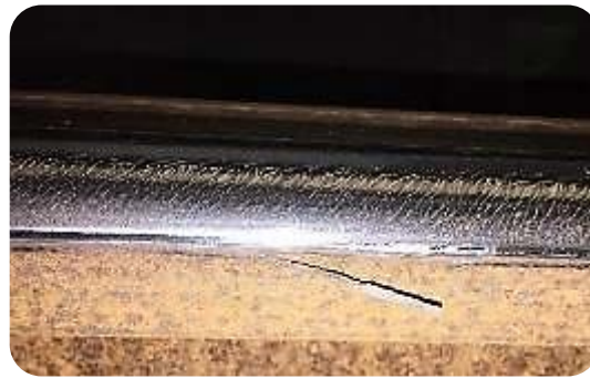
Shatter crack and head checking
