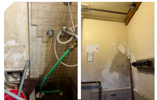
Deterioration of work spaces Cuyamaca College, F Building
