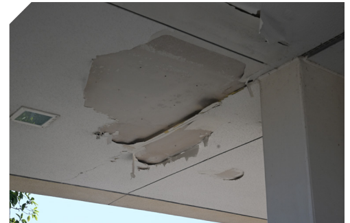
Leaking roofs Grossmont College
