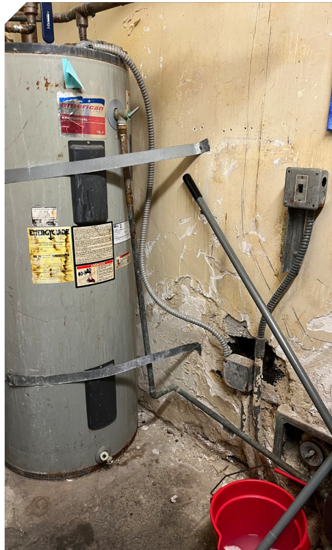
Aging water and electrical systems Cuyamaca College, F Building
