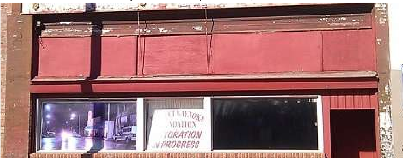
Building in disrepair, Photo Courtesy of: City of Warren
