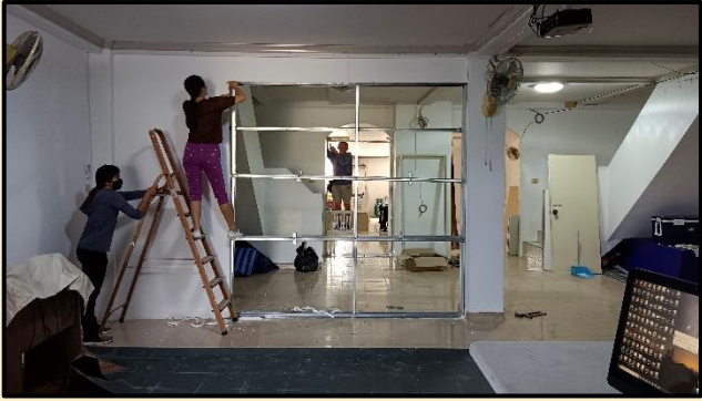
1. The renovation of our church building. We need more space for worship as we have more members.
